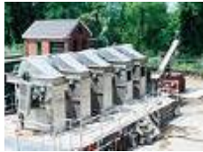
Screening/ Grit Removal
