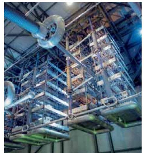
Efficient High-Voltage Direct-Current Transmission Systems (HVDC)
